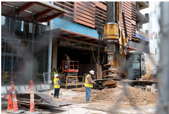
Construction work on 405 Colorado, developed by Brandywine Realty Trust. Ilana Panich-Linsman for The New York Times
